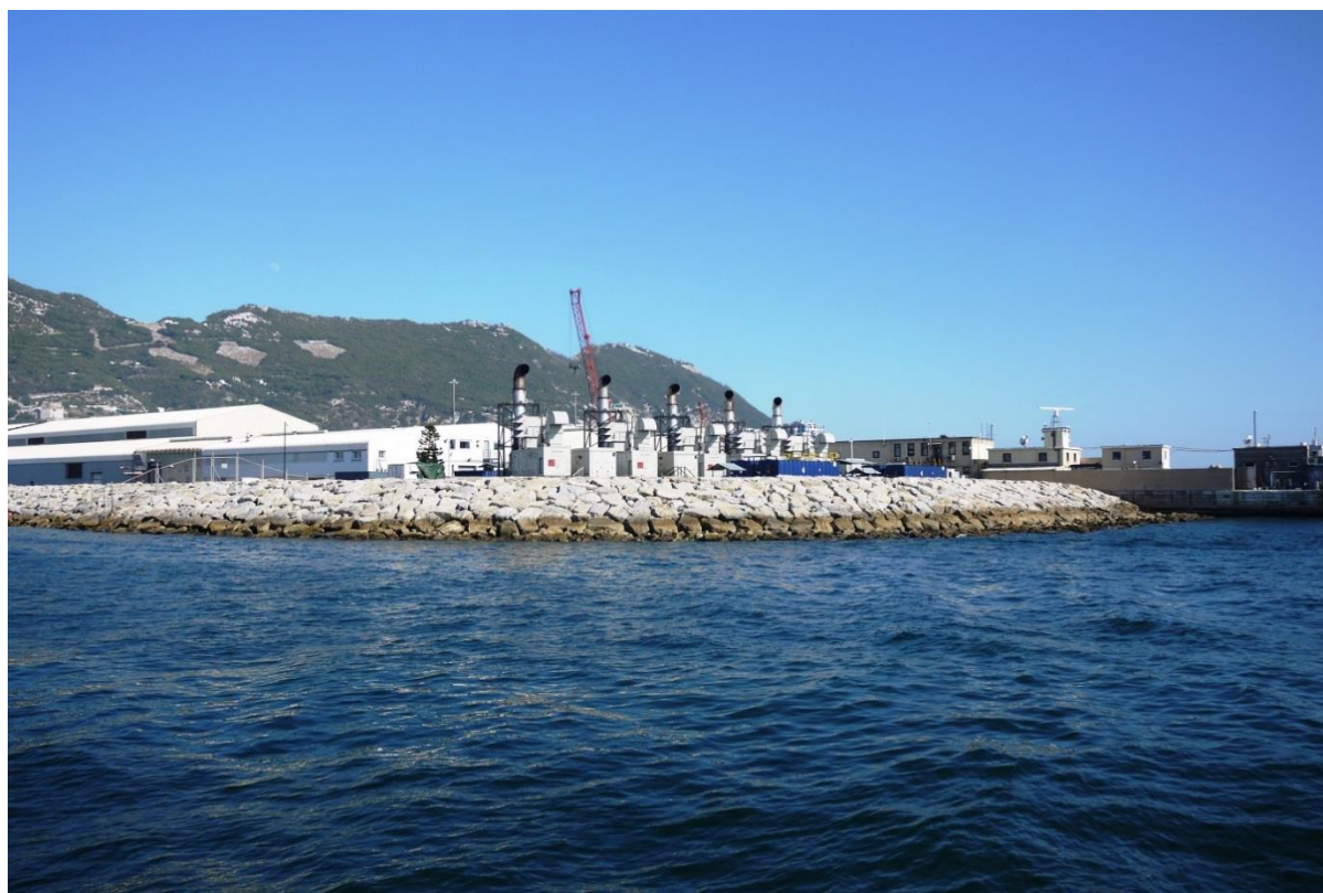
Figure 4-2: Turbines at North Mole
