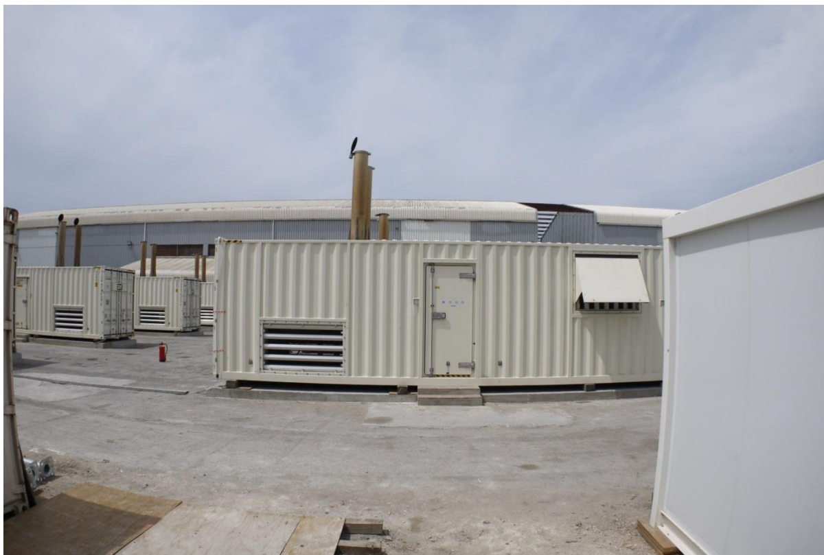
Figure 4-3: New skid-mounted generators at North Mole (2014)
