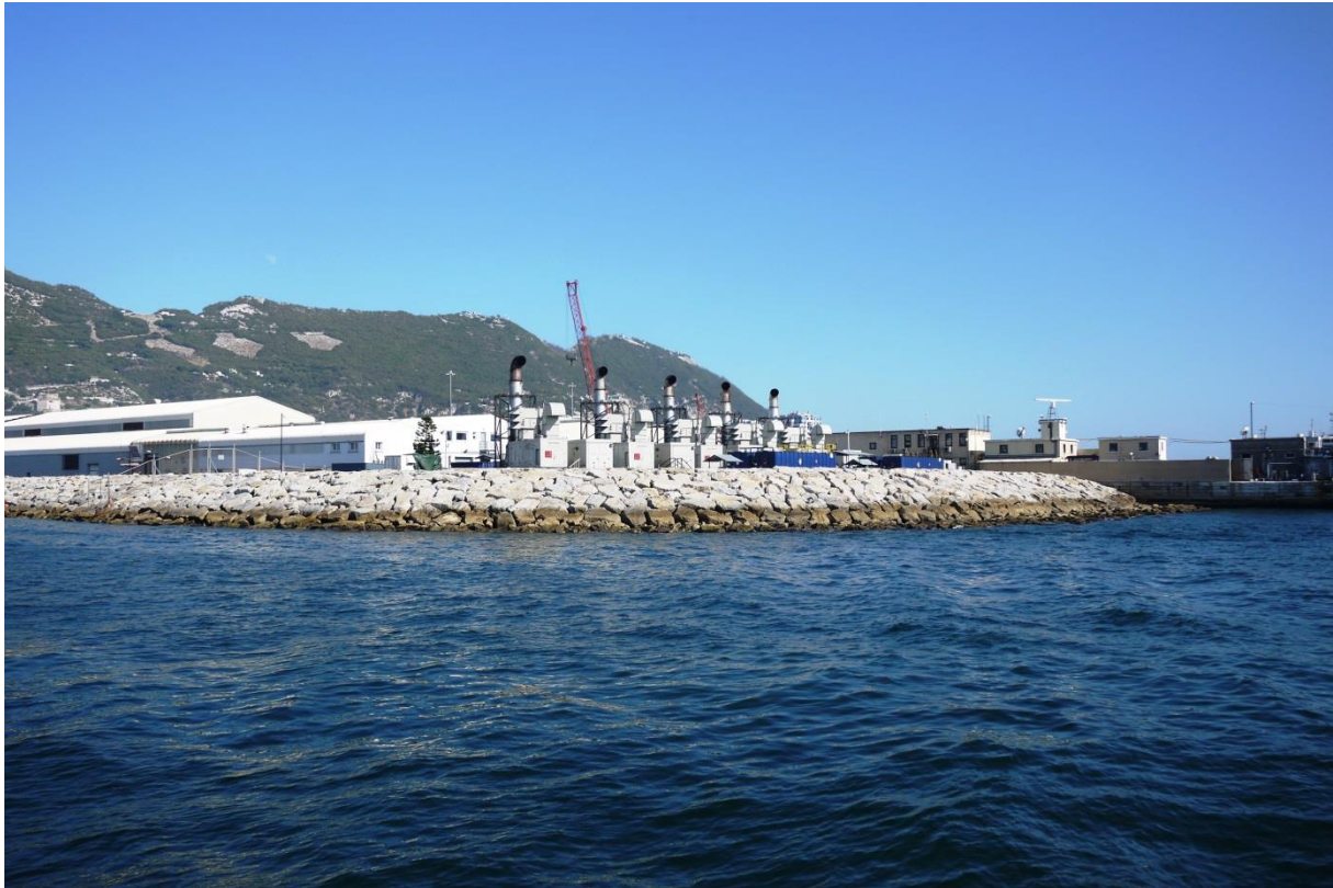
Figure 4-3: Turbines at North Mole
