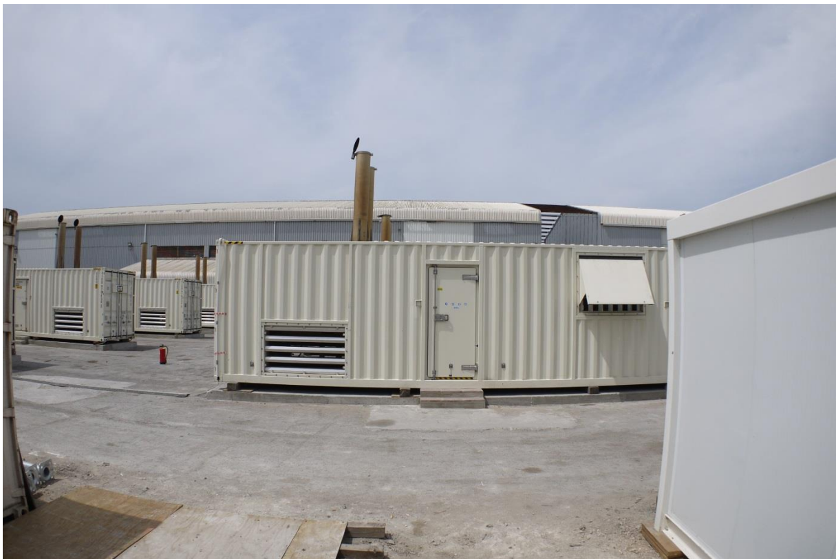
Figure 4-4: New skid-mounted generators at North Mole (2014)
