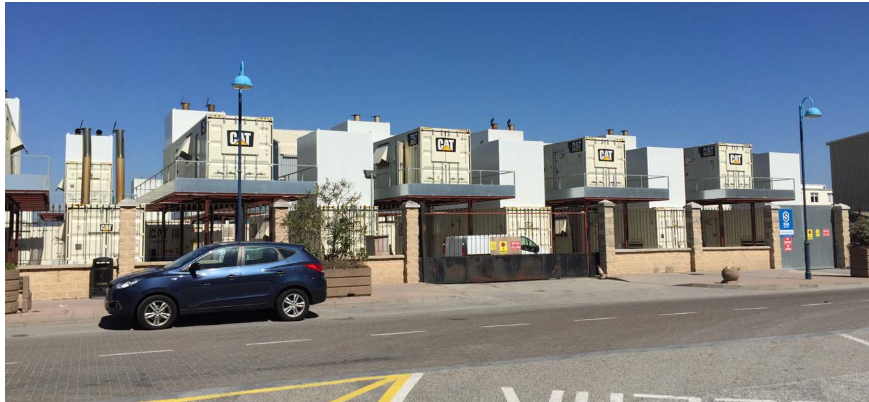
Temporary Caterpillar Generating Units on North Mole Road
