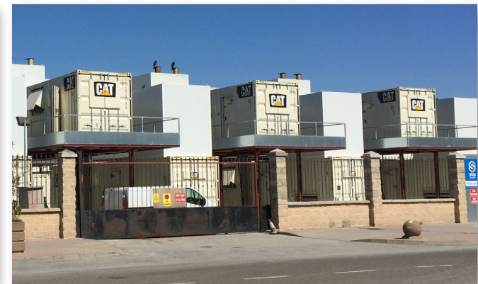
TEMPORARY CATERPILLAR GENERATING UNITS ON NORTH MOLE ROAD
