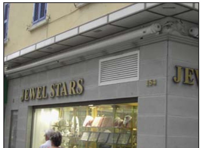
Air condition units recessed within elevation.
