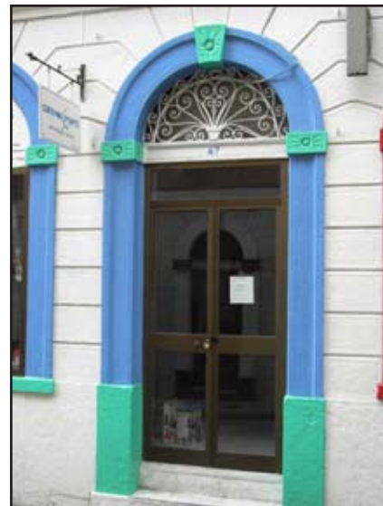
Inappropriate painting of original stone features
