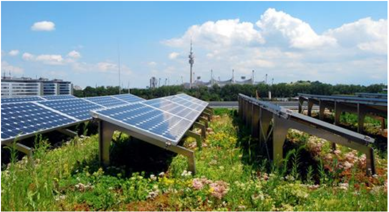
Greenscape green roofs with solar panels
