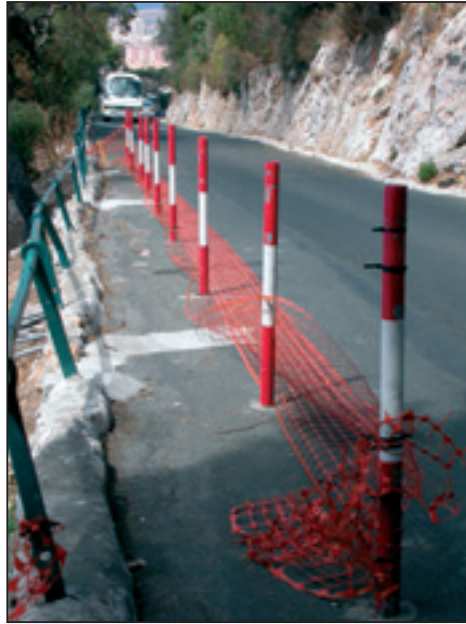
Figure 3. Road works – this makeshift barrier has been present at St. Michael's Cave for over a year, where nothing has been done to improve the situation.
