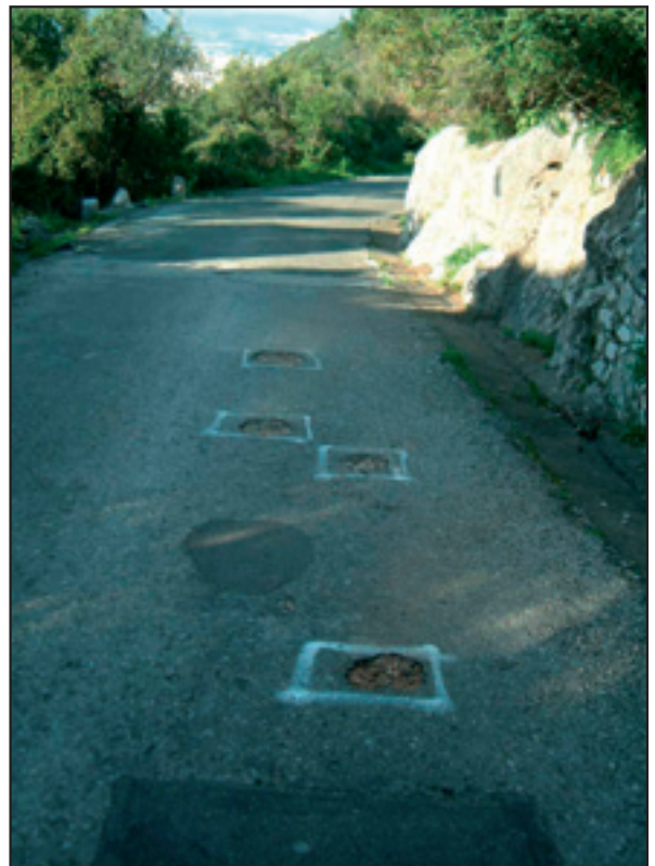
Figure 4. Potholes along Queen's Road remained marked by a white or yellow, square perimeter for a long time before being filled.
