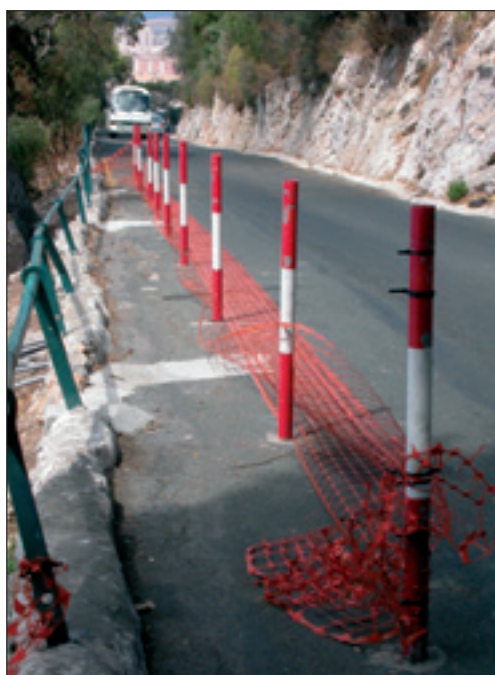
Figure 5. Road subsidence at the top of Cave Branch Road.
