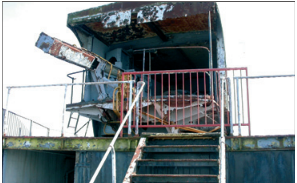
Figure 5. Lord Airey's Battery rusting away.
